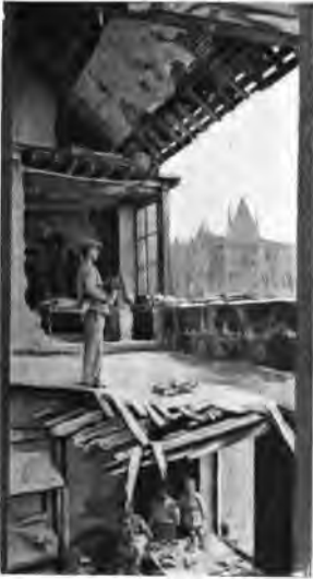
THE FIRST AND SECOND STORIES OF A HOUSE IN THE RUE D'ANJOU, AFTER THE BURSTING OF AN 8-IN. SHELL
