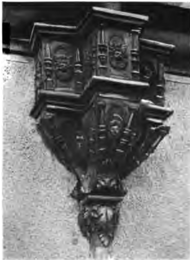
ORNAMENTAL RAIN-WATER PIPE-HEAD OF LEAD UNDER THE ROOF OF THE HOSPICE NOËL CAQUÉ (see p. 97)
