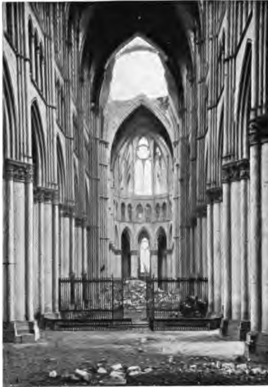
THE VAULTING OF THE CHOIR FELL IN ON THE HIGH ALTAR
